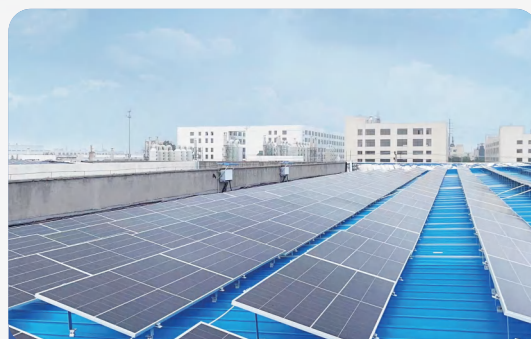
1.2MW Rooftop PV Plant in Jiangsu, China (XG100KTR)
