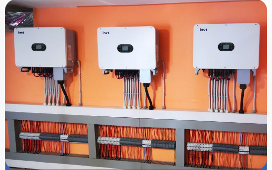
180kW Rooftop PV Plant in Lebanon (XG60KTR)
