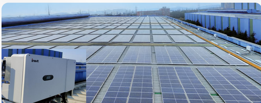
13.86MW Rooftop PV Plant in Hubei, China (XG136KTR-X)
