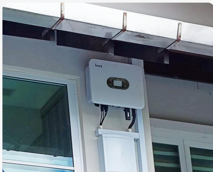
12kW Solar System in Malaysia (XG12KTR)
