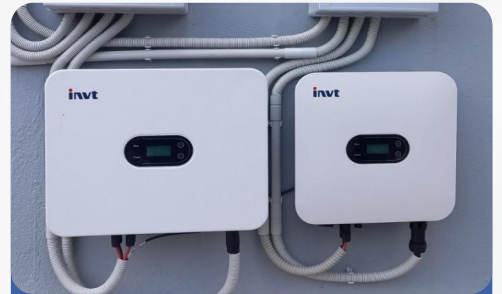
16kW Solar System in Greece (XG6KTL, XG10KTR)
