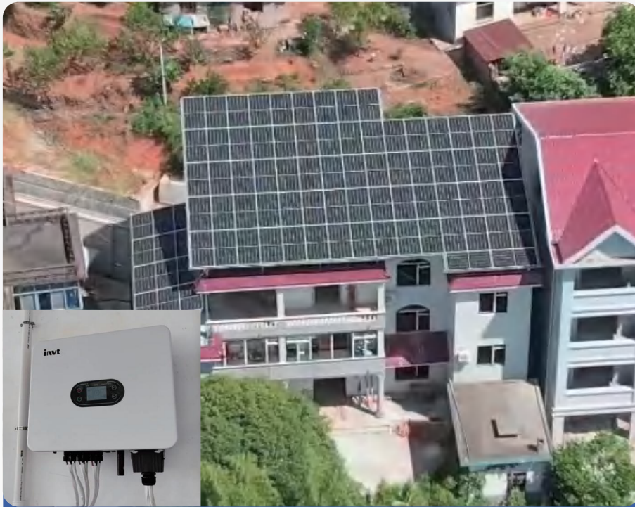
40kW Solar System in Jiangxi, China (XG40KTR)
