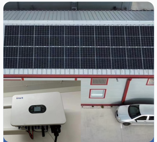
25kW Solar System in Slovakia (XG25KTR)
