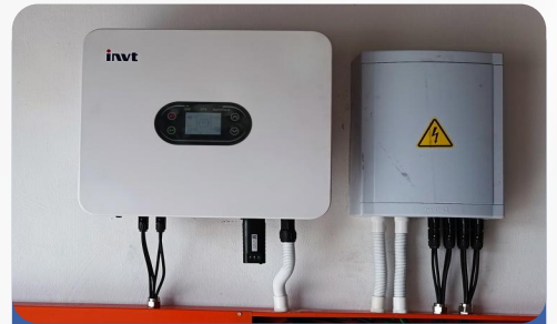
25kW Solar System in Malaysia (XG25KTR)
