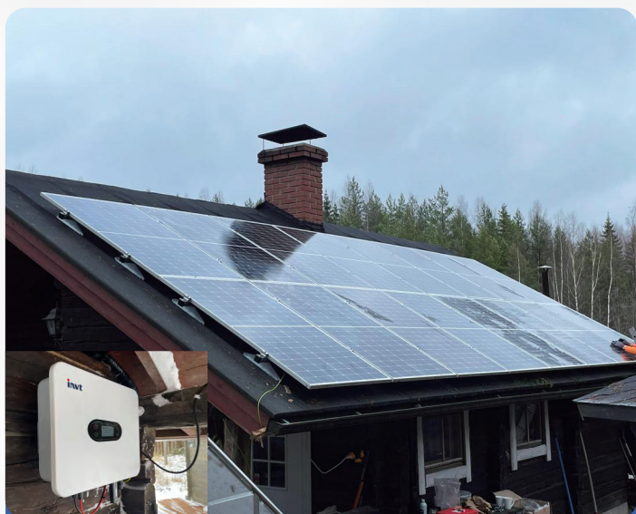
8kW Solar System in Finland (XG8KTR)
