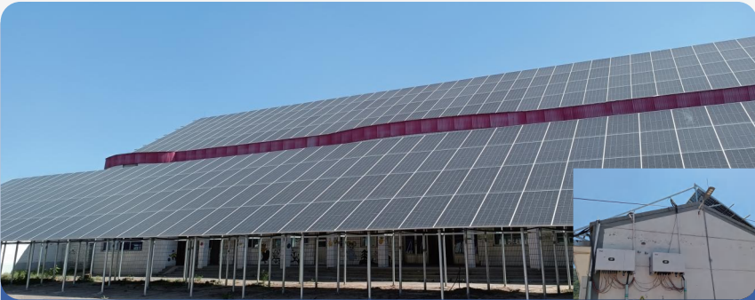
800kW Rooftop PV Plant in Shanxi, China (XG110KTR)
