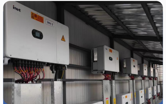
2MW Rooftop PV Plant in Türkiye (XG110KTR)
