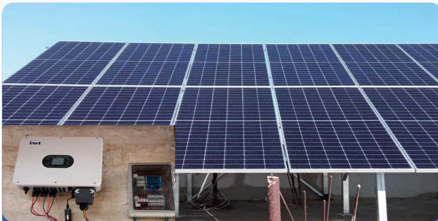
30kW Solar System in Israel (XG30KTR)
