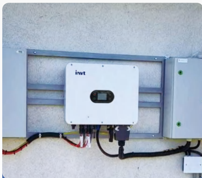
30kW Solar System in Serbia (XG30KTR)
