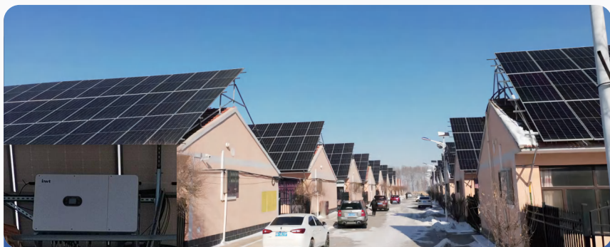
11.6MW Rooftop PV Plant in Hebei, China (XG110KTR, XG60KTR)
