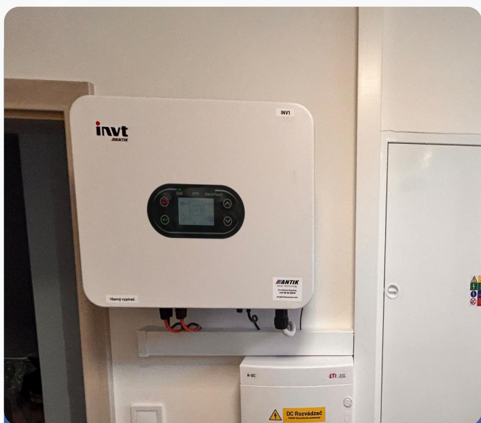
10kW Solar System in Slovakia (XG10KTR)
